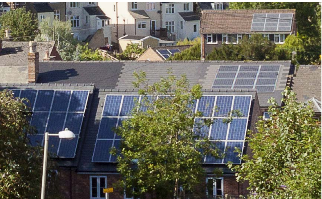
Domestic photovoltaic panels in Stroud.
